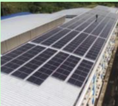
Figure 2: UniCAM Main Campus with rooftop solar installation
